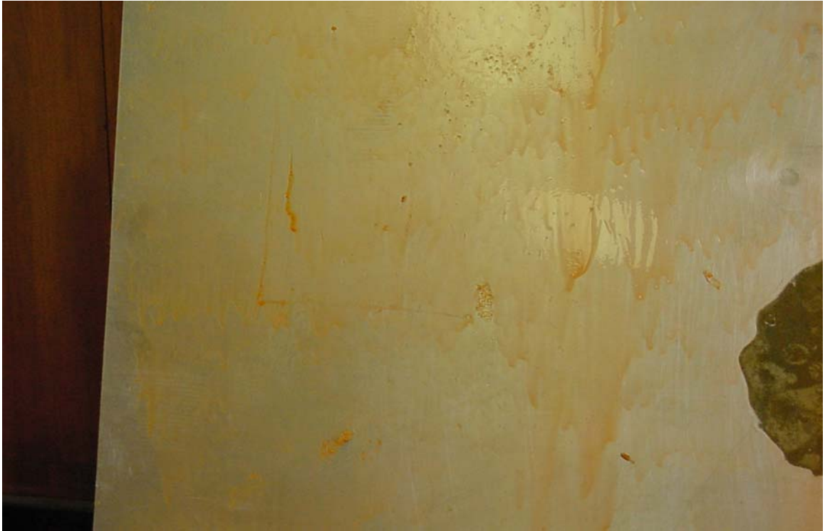
Figure 1.5-16 Unacceptable Coating Color Concentration.
