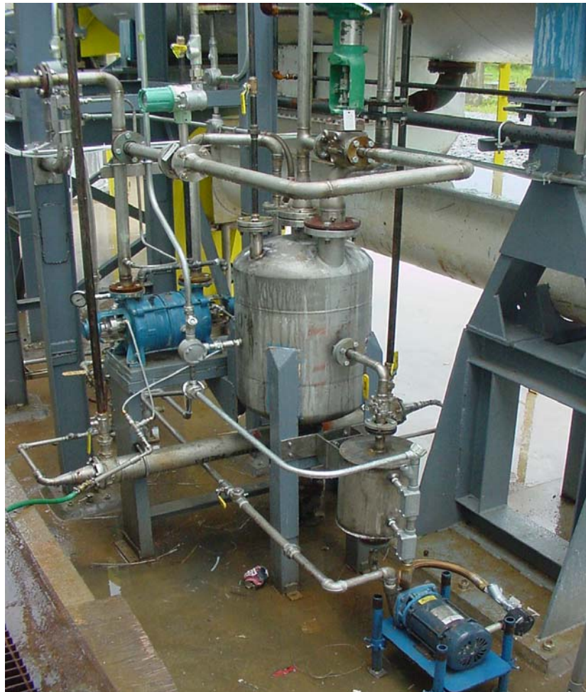
Figure 4.2-5 Vacuum Pump System.
