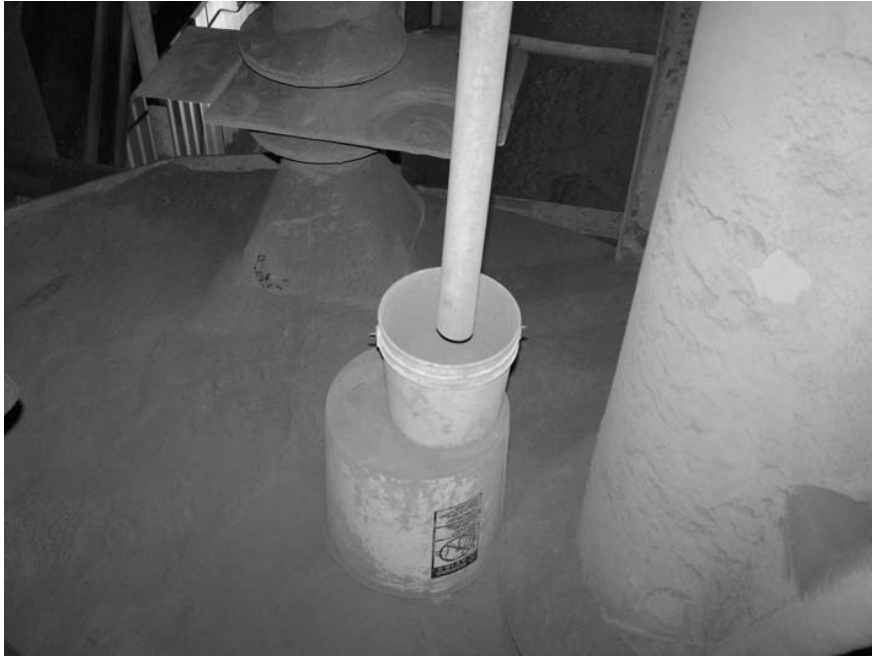
Figure 3.14: Portland cement sampling point
