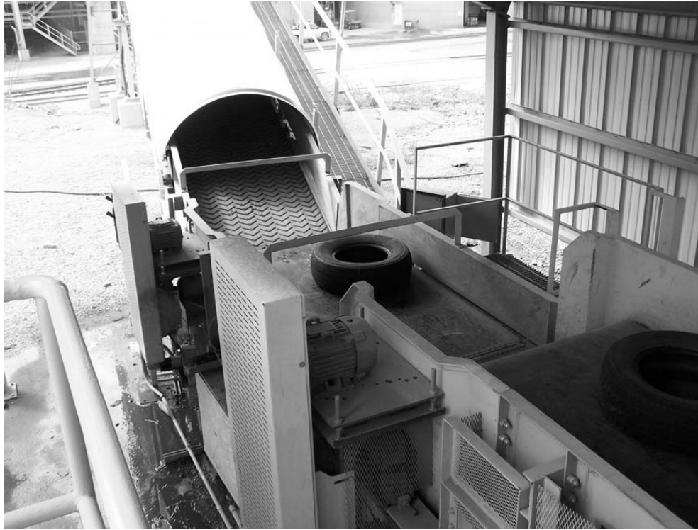
Figure 3.7: Tires conveyed to kiln
