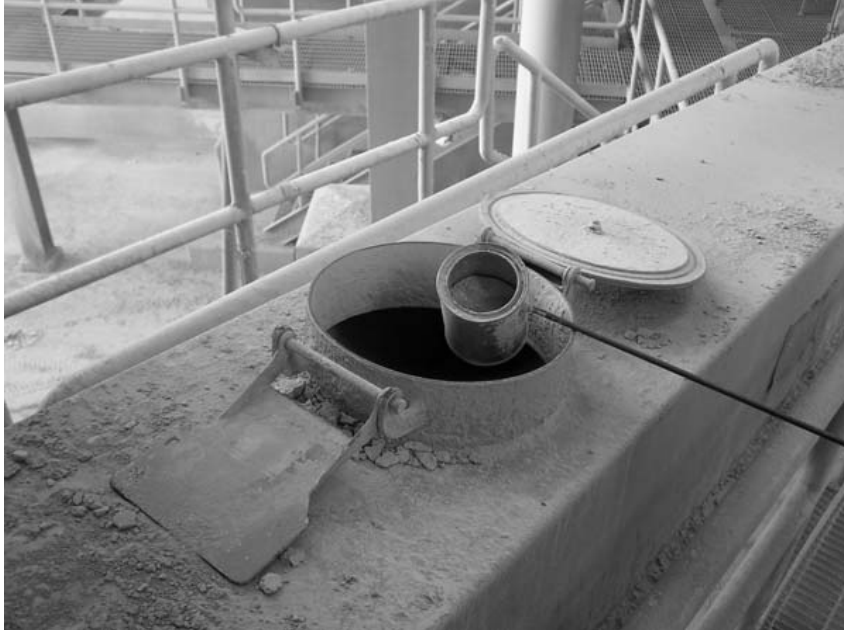
Figure 3.5: Kiln feed sampling point
