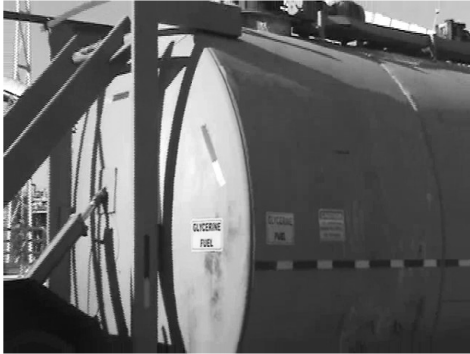
Figure 3.11: Glycerin storage tank
