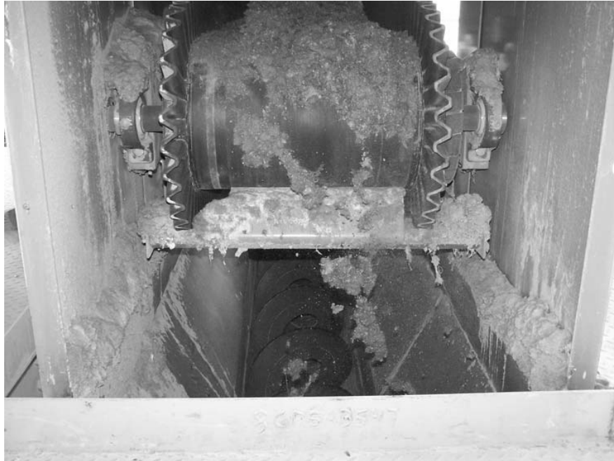
Figure 3.9: ASF/waste plastics conveyer and injection system
