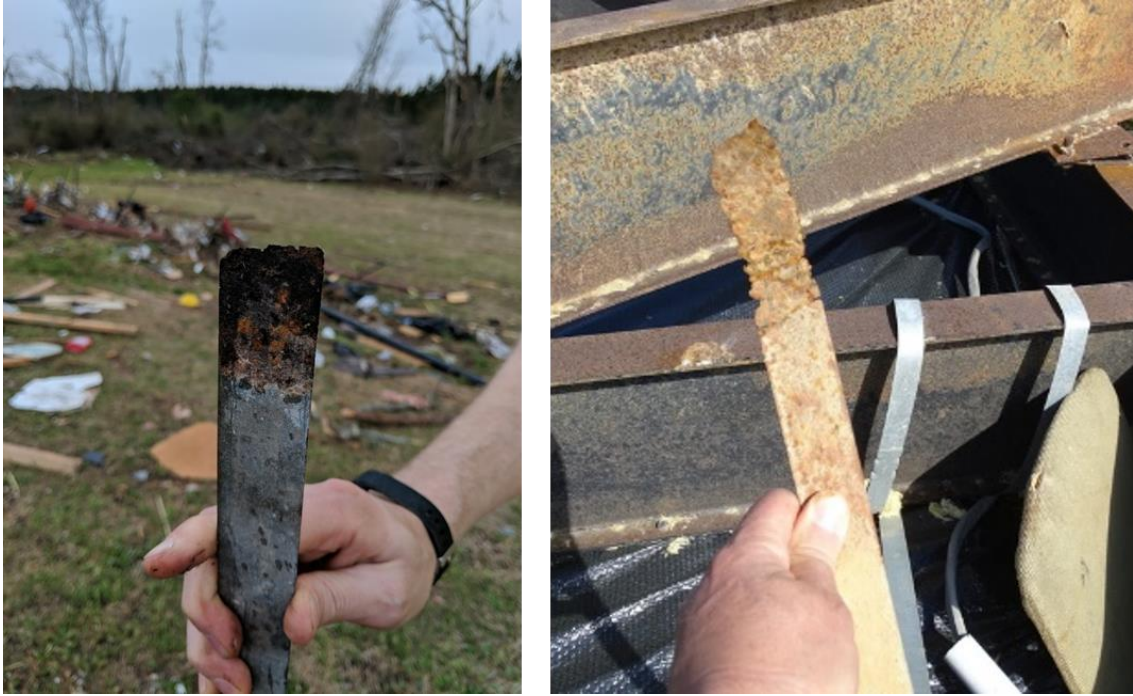
Figure 4-8. Strap failure due to corrosion
