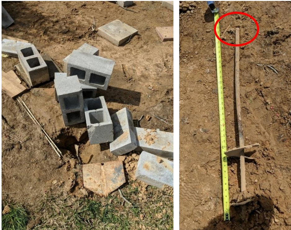
Figure 4-22. Anchor pullout (left) and detachment of the anchor head (right)
