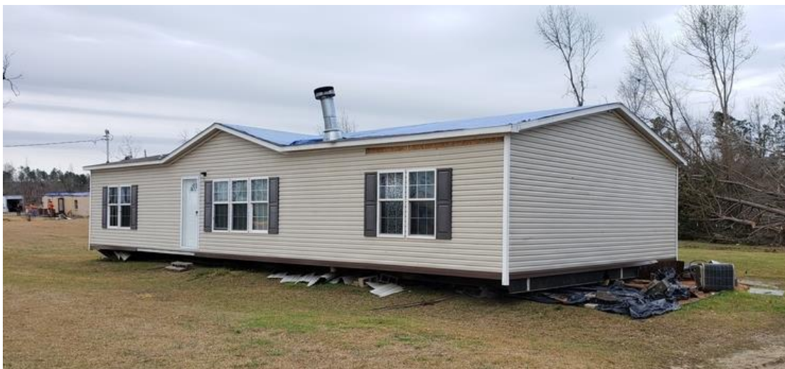
Figure 4-5. Sliding off the home off the foundation
