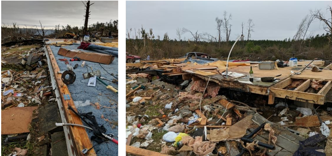
Figure 4-4. Failure of the wall-to-floor connection
