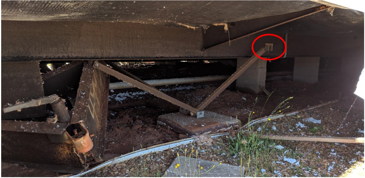
Figure 4-19. Connection failure of an impacted pan system
