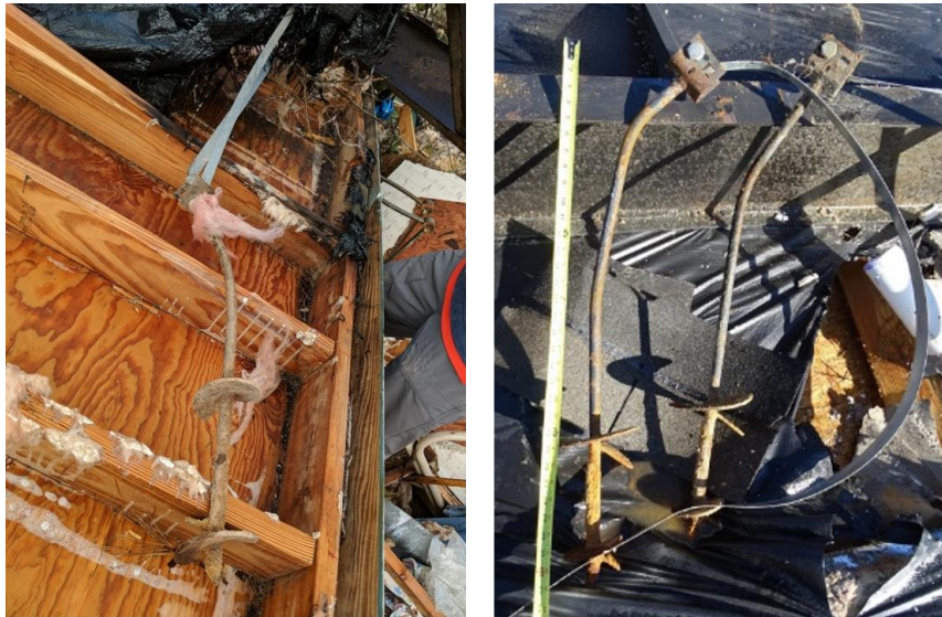
Figure 4-9. Anchor pullout failure
