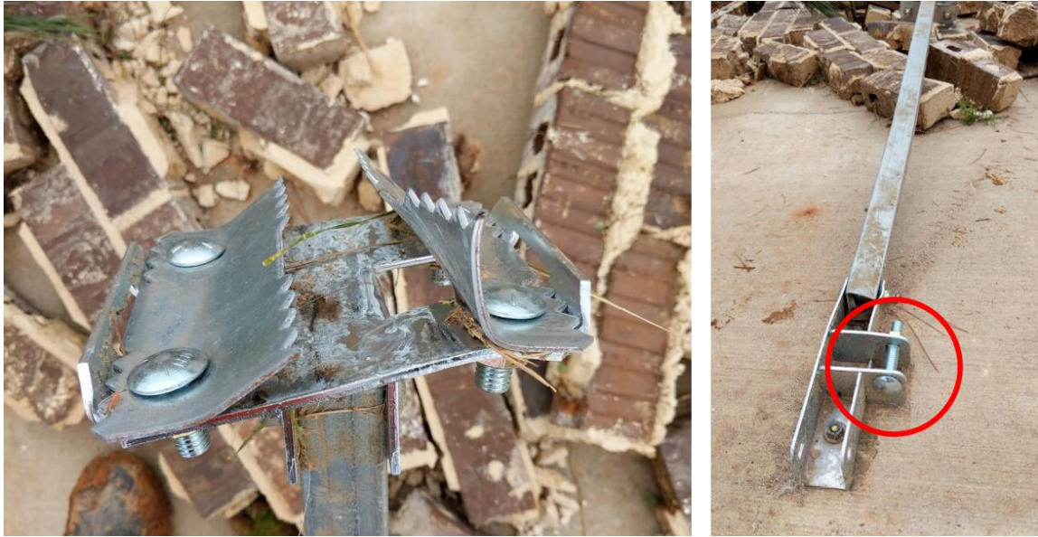
Figure 4-12. Failure of pan system struts at the I-beam (left) and the foundation attachment (right)
