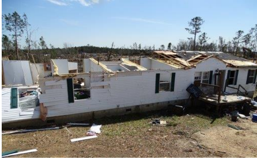
Figure 4-3. Failure of the roof-to-wall connection
