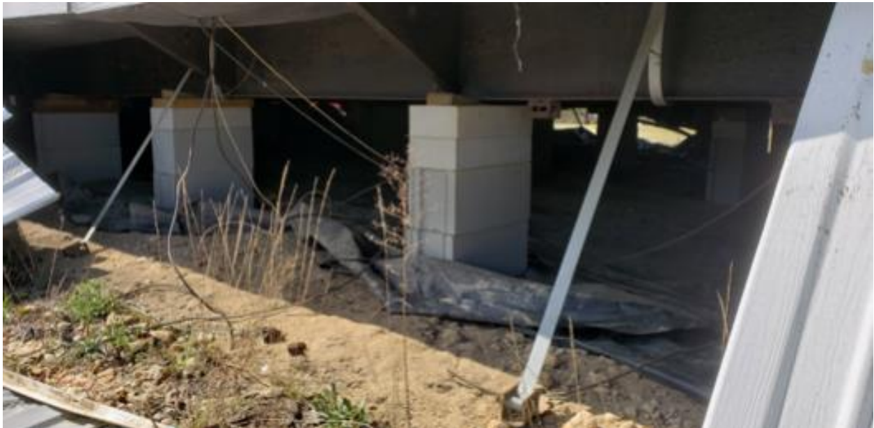
Figure 2-2. Typical diagonal tie-down straps, attached to the near I-beam.
