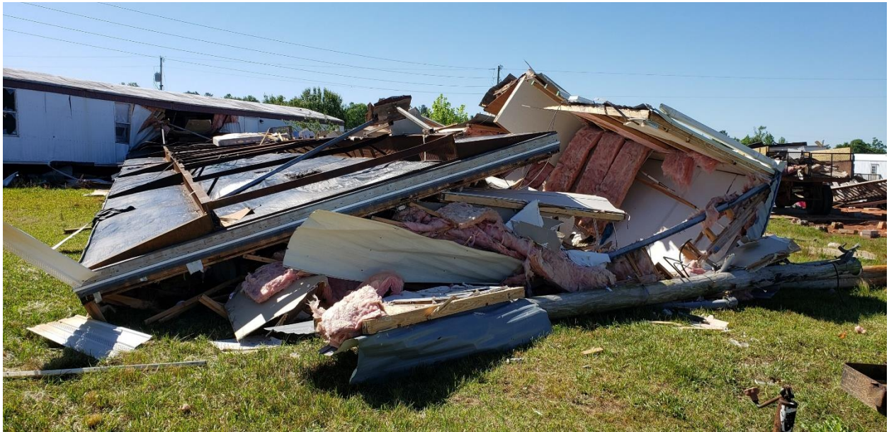
Figure 4-20. Lofting of a pan system leading to destruction
