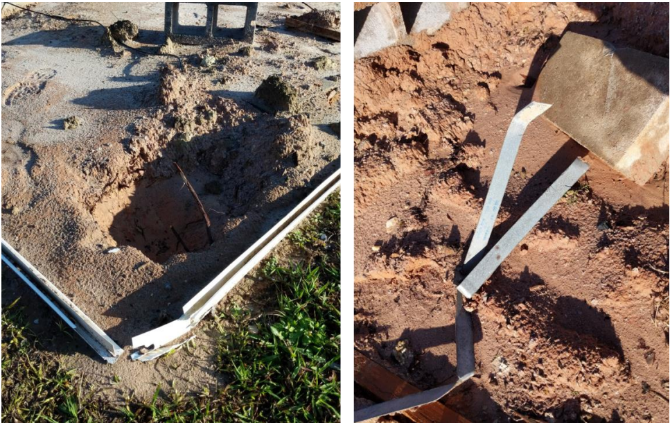
Figure 4-16. Anchor pullout (left) and strap failure at the I-beam (right)
