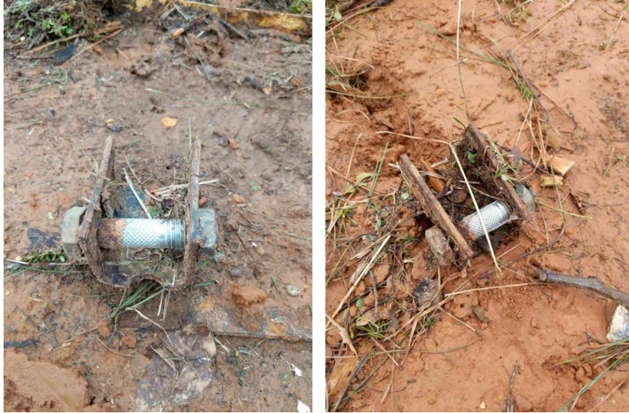
Figure 4-11. Evidence of straps pulling out of anchor heads
