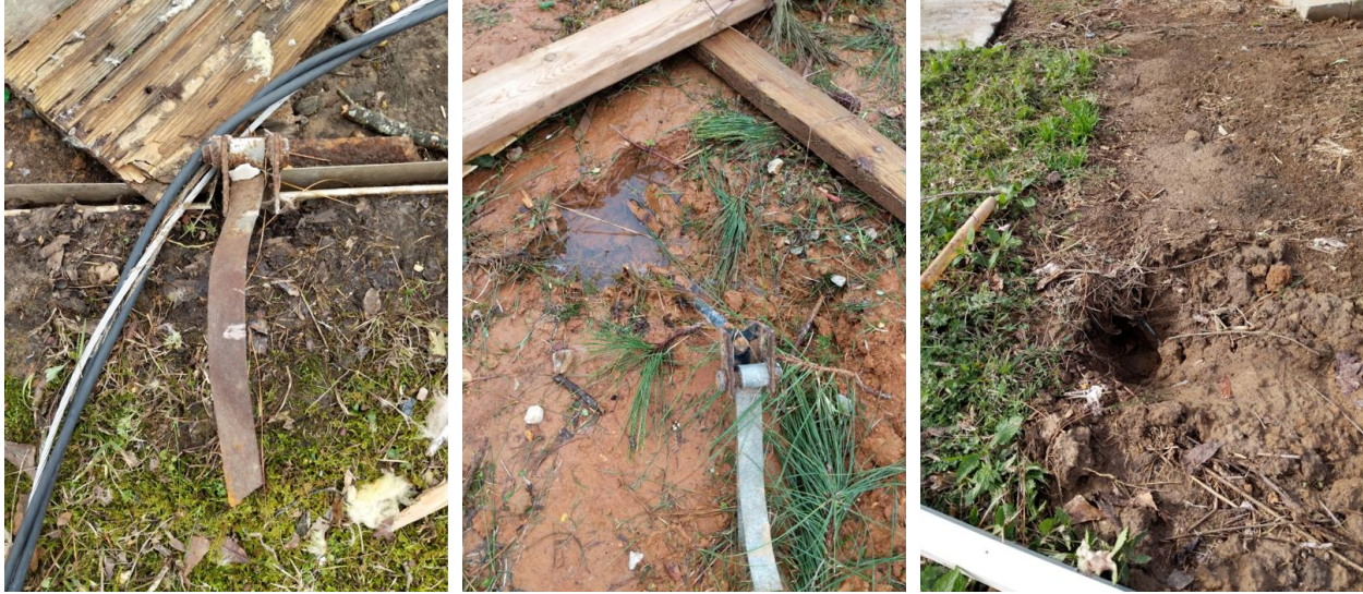
Figure 4-13. Corrosion failure (left), anchor deflection (middle), and anchor pullout (right)
