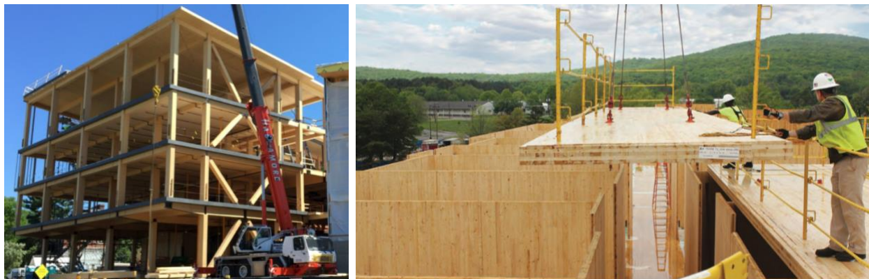
Figure 2-18: Mass timber construction. Examples of post and beam construction (left) (LWA 2022) and panel construction (right) (WoodWorks 2016).
