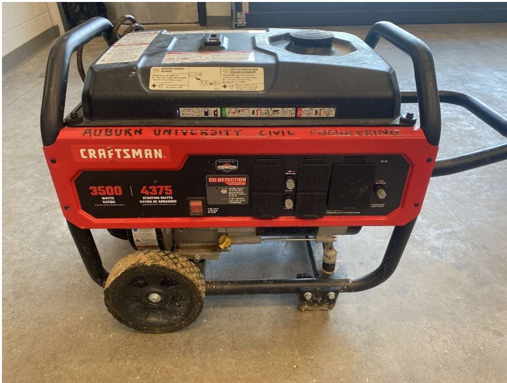
Figure 3-8: Generator used to provide power to SIC Curing Box
