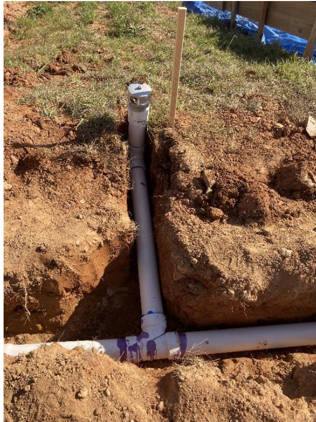
FIGURE 3.13: Supply Pipe Outlet.
