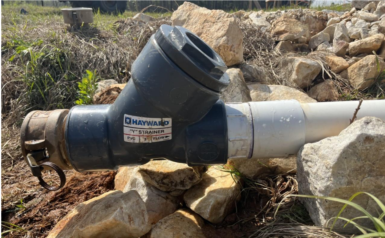
FIGURE 3.16: Supply Pipe Intake Debris Filter.
