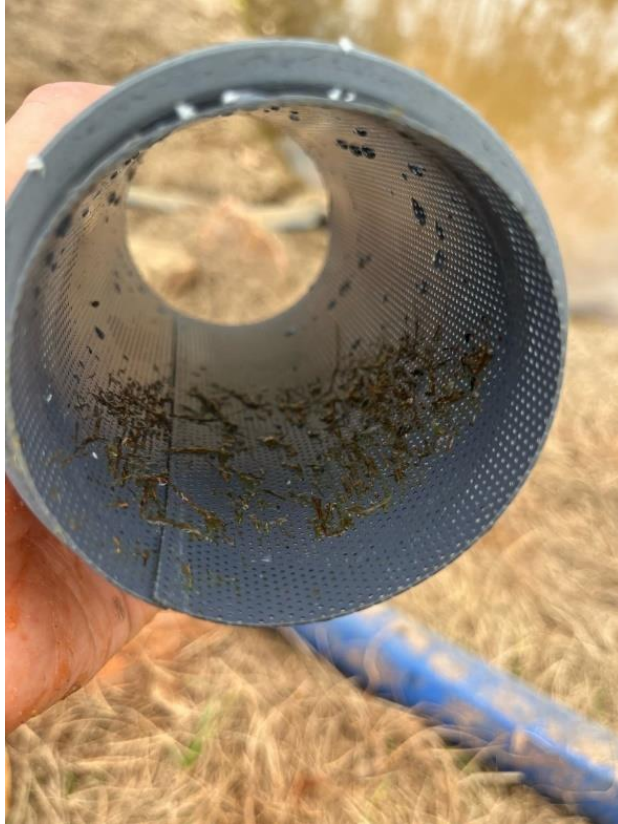
FIGURE 3.17 Debris Caught by Filter.
