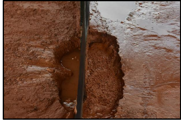
(b) trench failure
