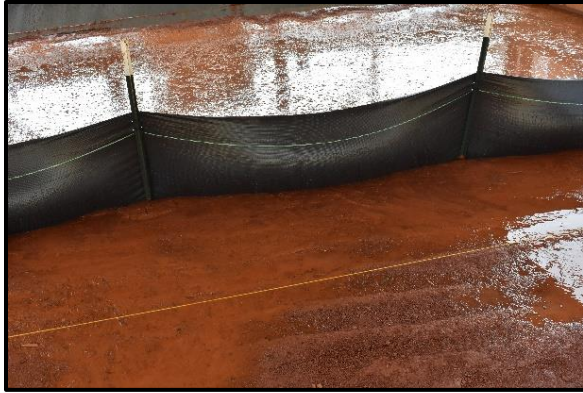
(a) undermining and sagging
