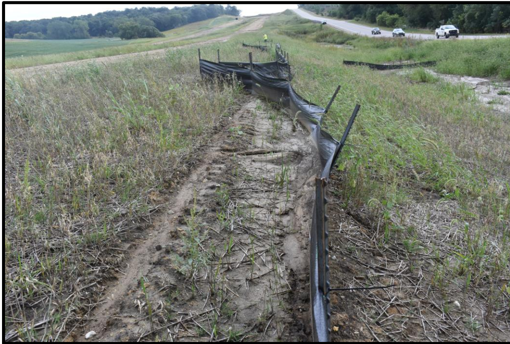
(a) Iowa standard silt fence installation experiencing excessive post deflection
