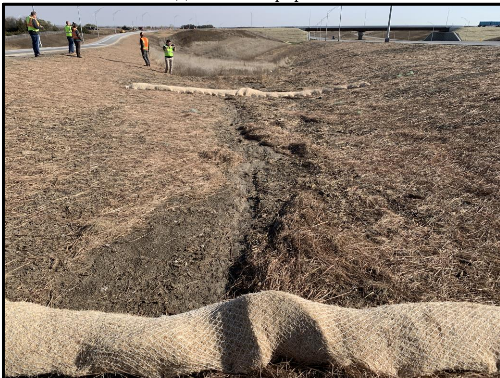
(b) wattles as ditch checks
