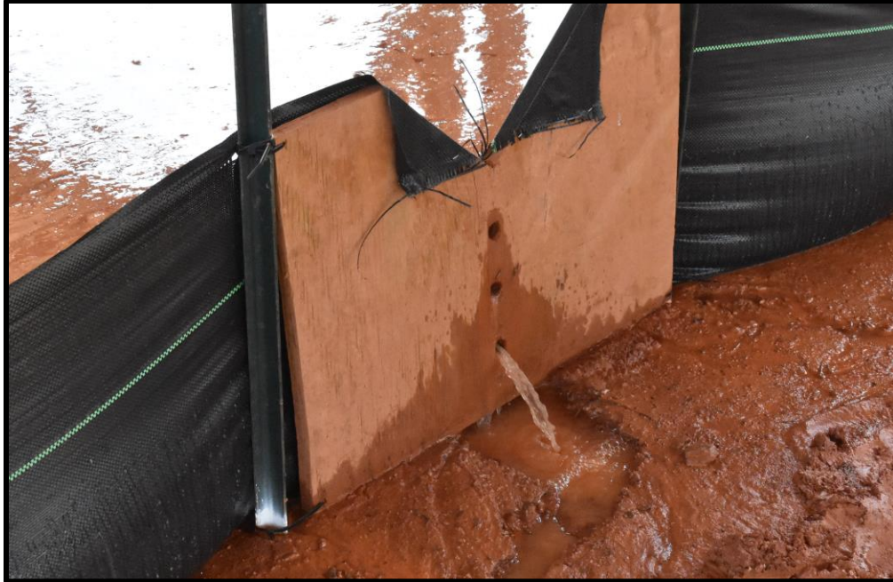
Figure 3.17 Scour Downstream of Dewatering Board Installation without Energy Dissipation Device
